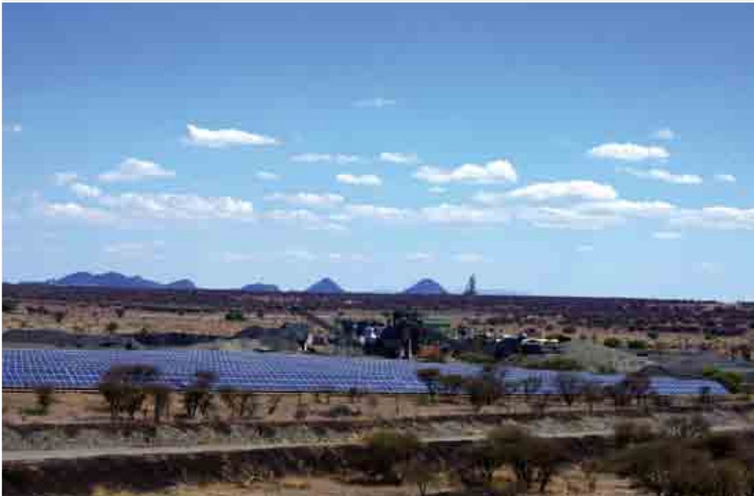
PV installation at Cronimet chrome mine, Limpopo
