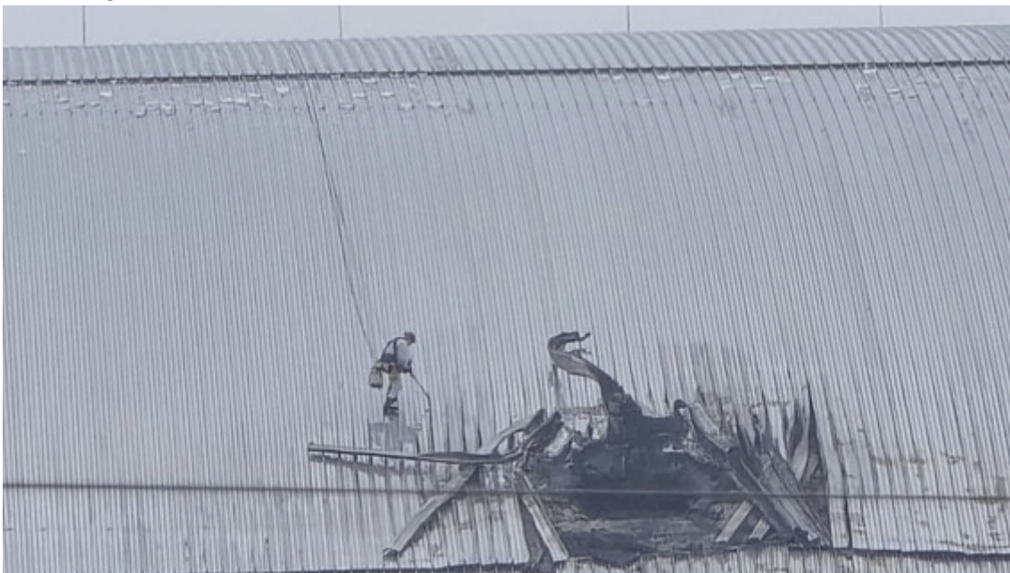
Photo 4: Chornobyl NPP damaged by the drone attack, February 2025. Source CHNPP 50
